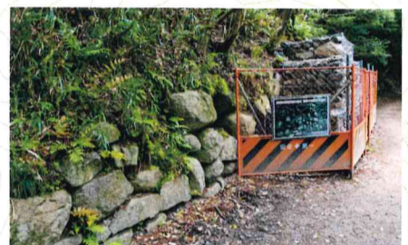
H Stone wall supporting the eastern slope of Division II This is the biggest one in Imori Fortress. It was reinforced with many gabions filled with stones at the bottom to refrain from destruction.
