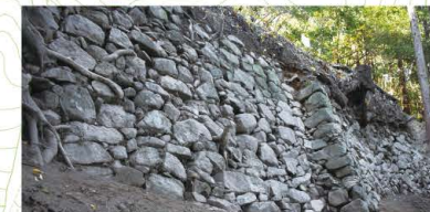
Biggest stone wall of this site at Division II. Corner area is provided for strength. This area is dangerous and is currently off-limits.
